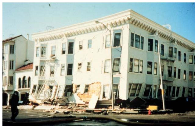
Figure 2 - Collapse building SE corner Jefferson and Divisadero, next day (Photo: Scawthorn, 1989)
